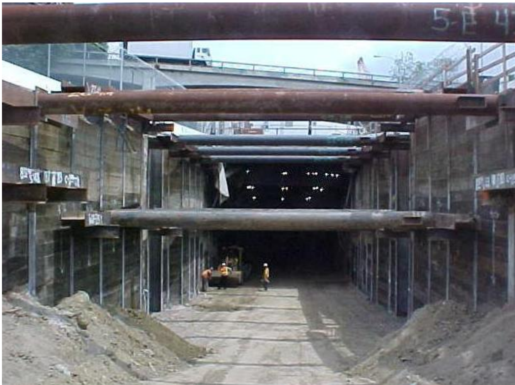
Gold Line Eastside Extension – West Portal entrance Gold Line Eastside Extension – excavation of utility trench under US 101
